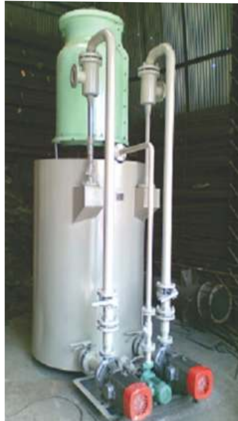
Solvent Recovery at Praveen laboratories pvt. ltd.- surat
