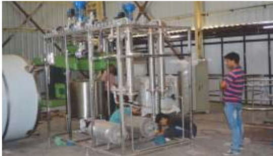
CIP High Pressure Water Distribution Skid
