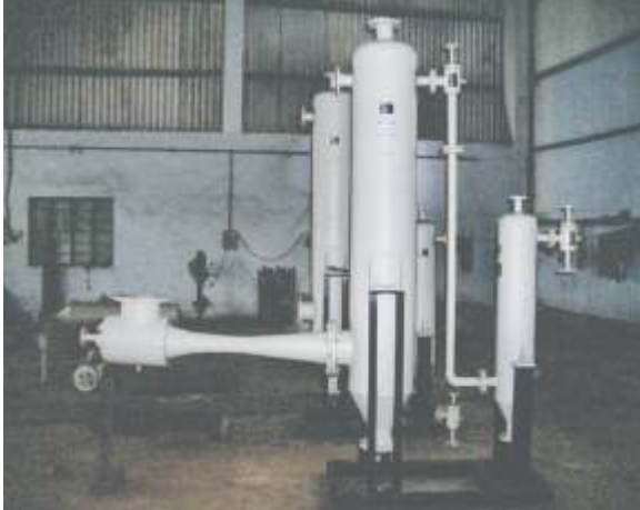
Double Stage Vacuum Booster (edible oil refinery)
